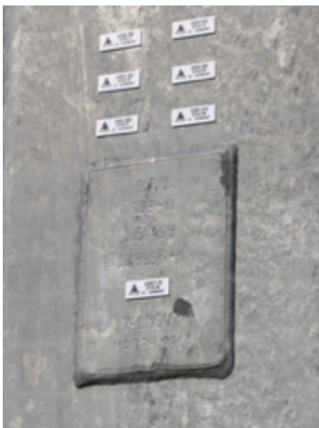
Secondary RFID tags for arms. Enables ground survey of arms attached to structure.
