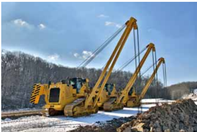
The PL83 pipelayer has a lift capacity of 170 000 lb (77 111 kg) and, like the PL87, meets the unique demands for big inch pipework in varied climates.
