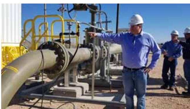
Figure 5. Injection point exiting pump station.
