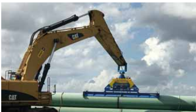
A Vacuworx RC 25 vacuum lifting system joined with a CAT 385 excavator handles 42 in. and 48 in. dia. natural gas pipe in south Texas.
