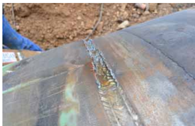
Figure 3. The greater control offered by the use of plasma rather the carbon arc to remove welds provides piece of mind for welders who no longer have to worry about blowing a hole through the pipe.
