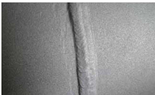
Figure 4. Was this area tested for residual salts?
