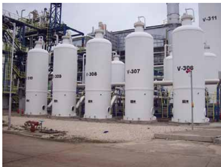
Figure 3. Hydrogen production plants: corrosion occurred because hydrogen bonded with carbon in the steel. Through fault detection analysis, MOL was able to get uptime back to 97%.
