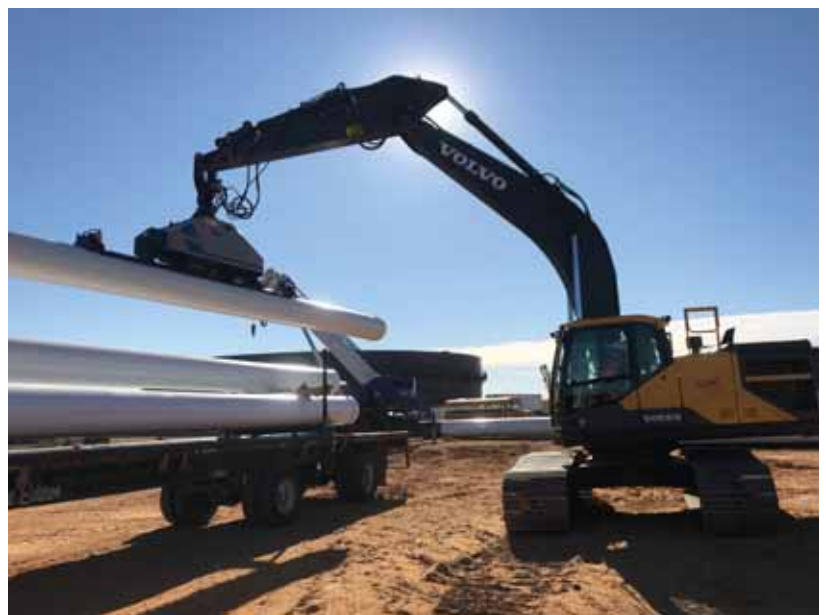
Contractor unloading and racking 20 in. OD x 40 ft long steel coated pipe with the PipeVac in Cushing, Oklahoma.
