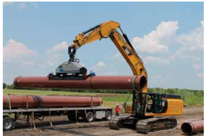
Contractor stringing 36 in. OD x 40 ft long steel coated pipe with the PipeVac in Venus, Texas.
