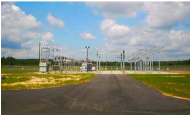
Figure 1. Dedicated compressor station electric substation.
