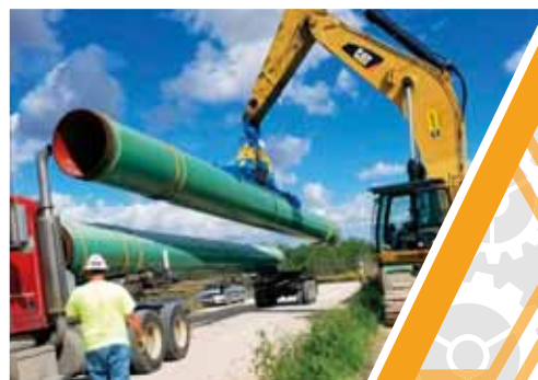
Vacuworx vacuum lifting technology offers a safer method of handling large diameter pipe in the field.
