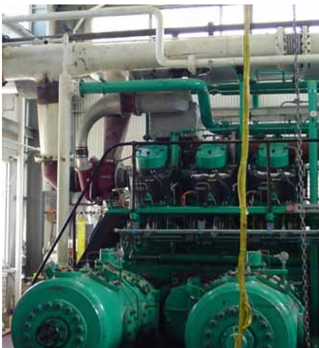
Figure 2. Reciprocating compressor installation.
